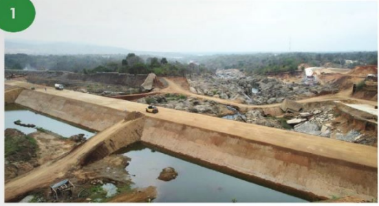
Picture 1: The completed cofferdam at Kapichira Dam, which stands at 148 metres above sea level
