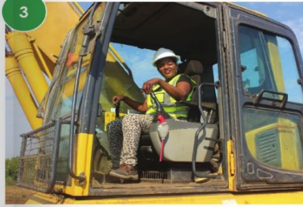
Picture 3: The SVTP has provided job opportunities to many people in the Shire Valley and other districts across the country including women like Aina Malonje, Operator at Sinohydro
