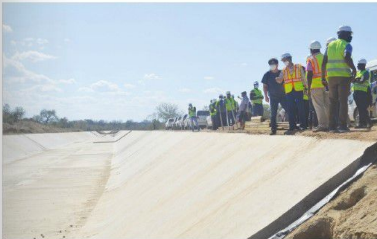
Work is progressing in spite of the Covid-19 pandemic which has slowed down works
