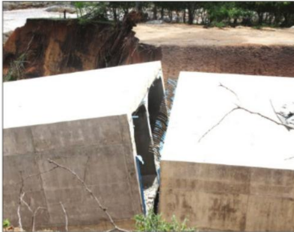
DAMAGED— Part of the structure— Picture by Eric Msikiti
