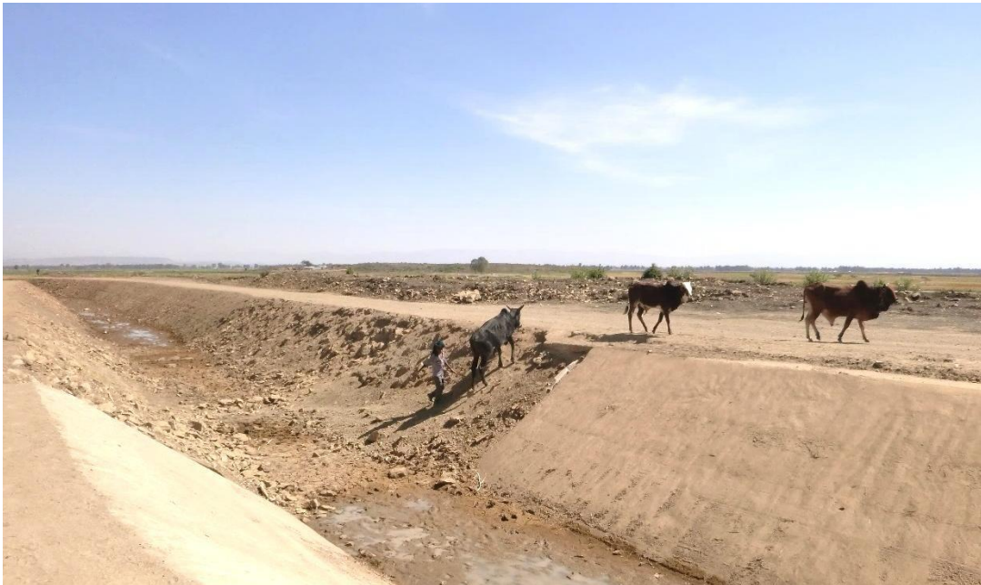
Figure 98: : Earth offers better grip than concrete (Source : BRLi, 2017)
