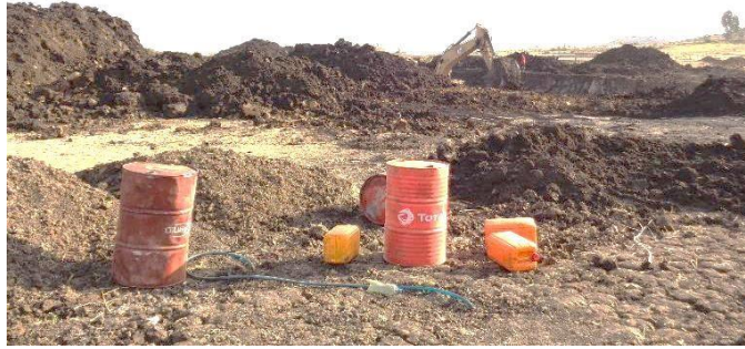
Figure 76: Poor oil management (Source: BRLi, 2015 )
