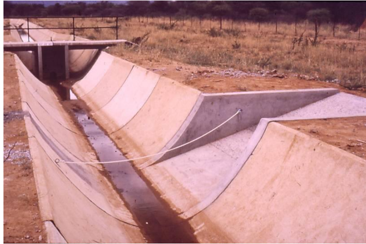
Figure 96: Inefficient escape structure (Source: Heyns, 2016 )
