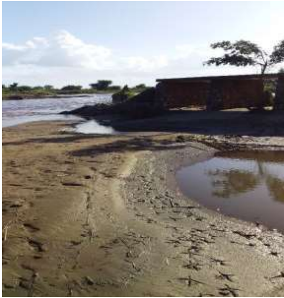
Figure 28: Washed away bridge on Mwanza River
