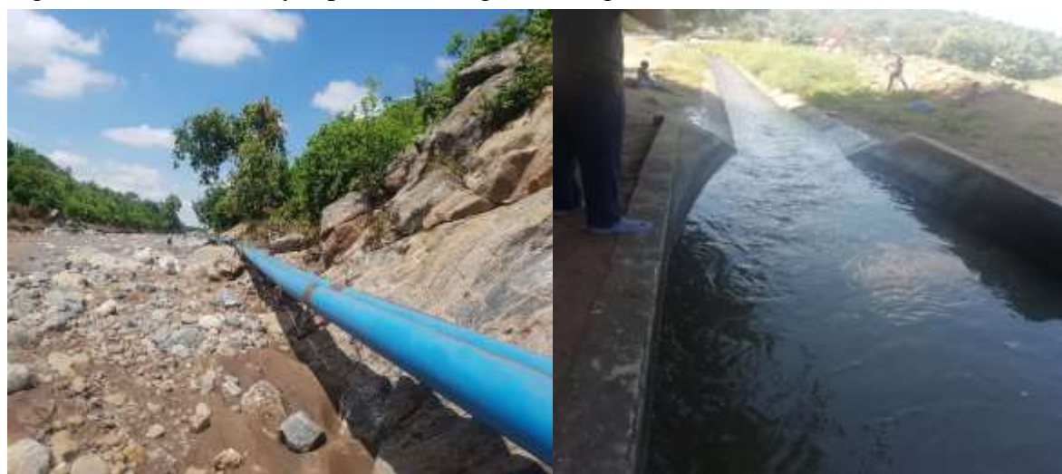
Figure 42: Washed away Pipes at Chilengo and Irrigation Canal at Phala
