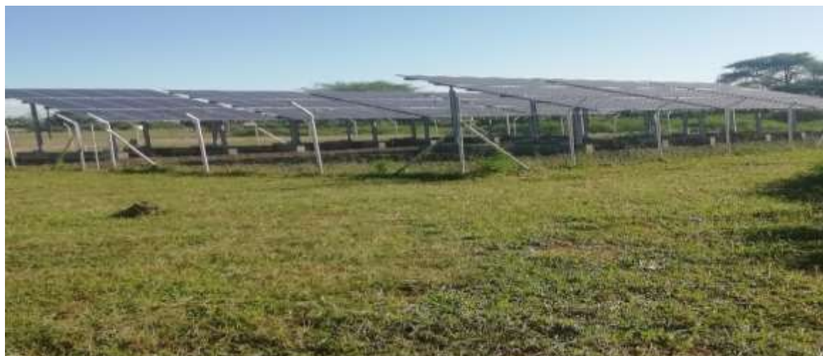
Figure 37: Solar Water Pumping at Chikwawa Boma
