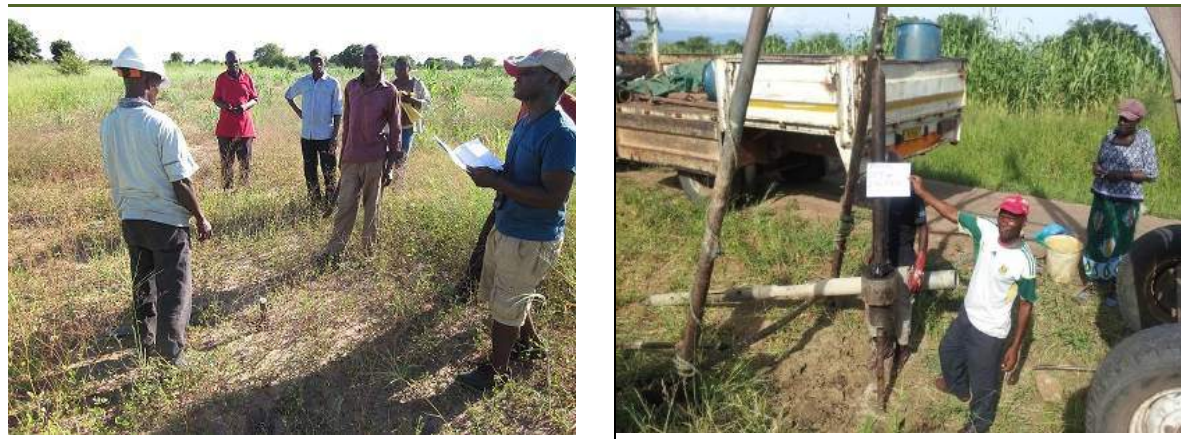
[Figure 2.3-2] Check of Drilling Point (left) and Percussive Drilling & Standard Penetration Test (right)
