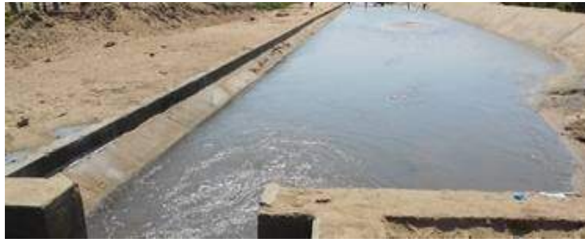
[Figure 3.10-3] Sand Trap of First Pump Station of Kasinthula
