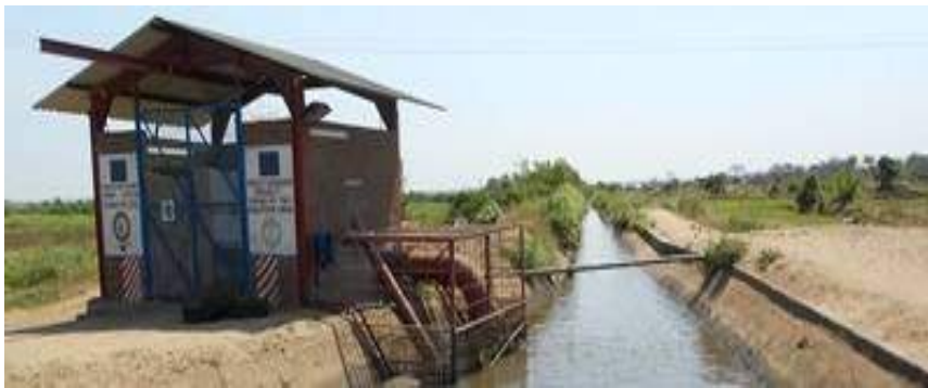
[Figure 3.10-4] Lined Canal and Second Pump Station of Kasinthula
