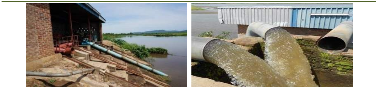
[Figure 3.10-2] First Pump Station of Kasinthula (Intake from Shire River)
