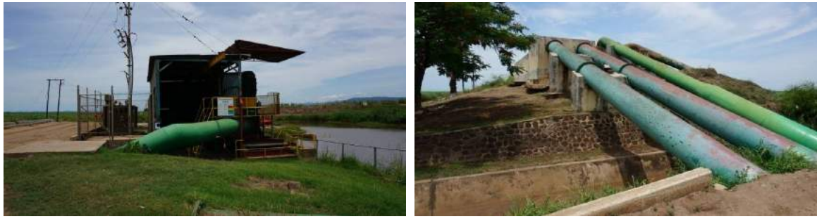
[Figure 3.10-6] First Pump Station (M1) of Nchalo (Intake from Shire River)
