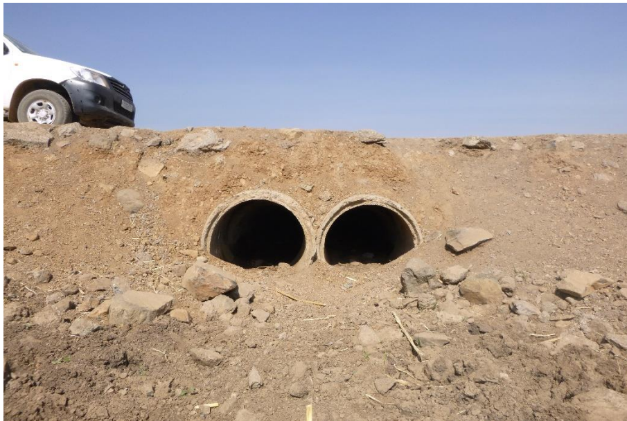
Figure 32 Inadequate culverts in an earth dike across a seasonal river
