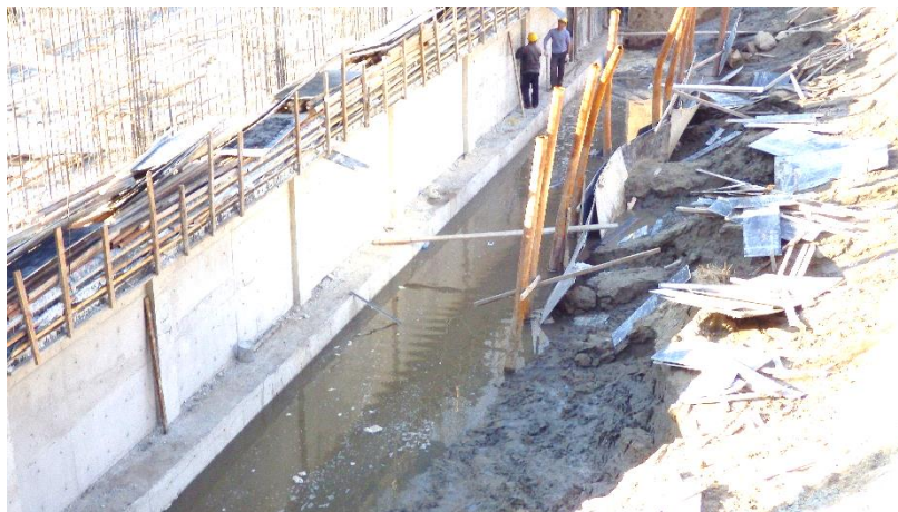
Figure 16 Working in damp condition around a pumping station
