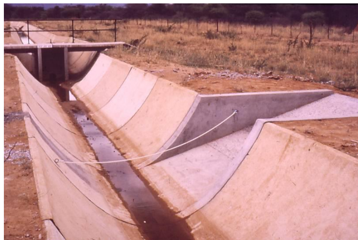
Figure 25 Inefficient escape structure
