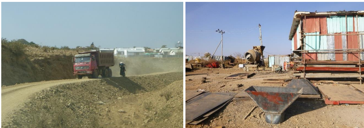
Figure 15 Trucks and pedestrians sharing construction roads & rubbish in construction camps
