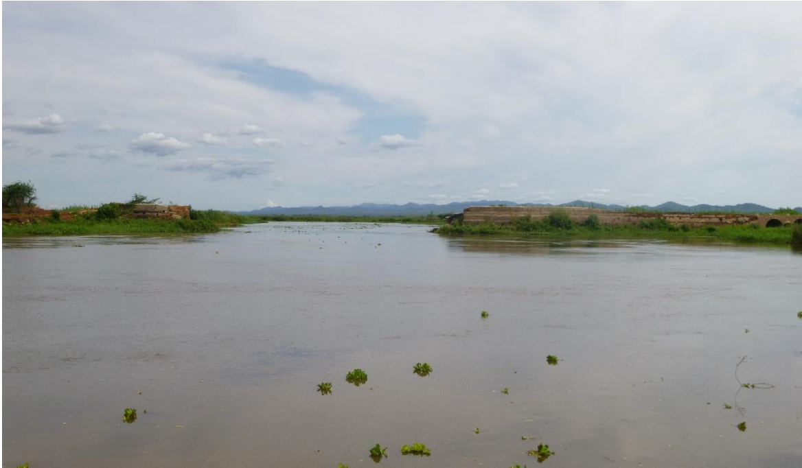
Figure 10 Broken Bridge over the Shire River at Chiromo
